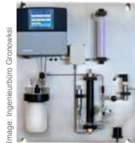
Measurement of degassed conductivity in power stations
